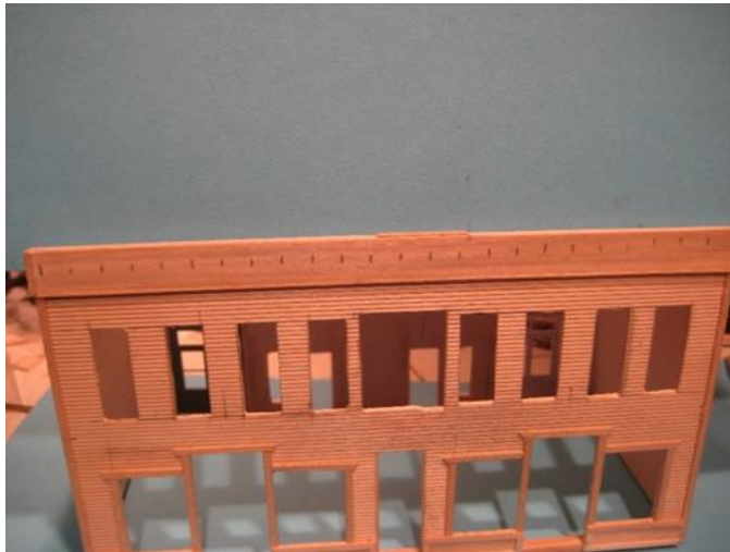
Fig. 18. Here the cornice is marked out for spacing of the decorative corbels.
