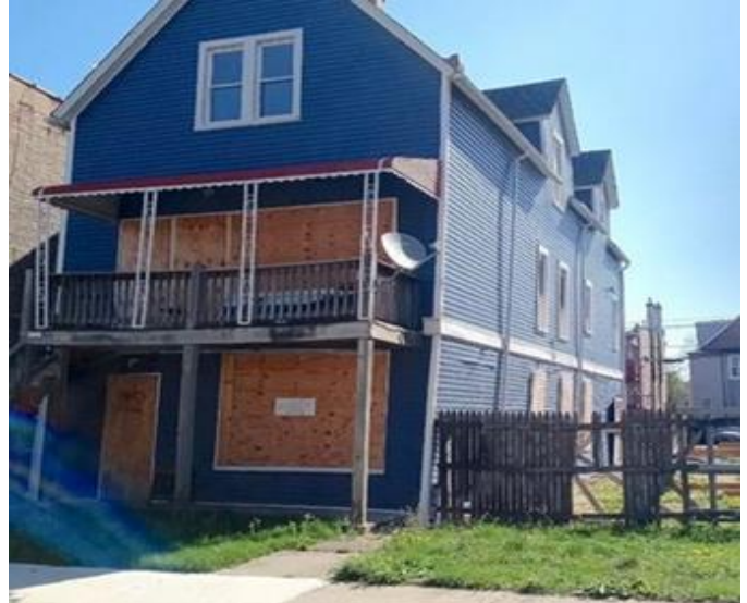
Fig. 4. Built circa 1900, this stack frame house shows the belt line between the first and second floors. It is balloon from the second floor and up. The failure in early stack frame was that the lower levels could sag out to one side or the other under the vertical load; as seen here in the white corner molding nearest the camera. The sag is particularly evident as the far end of the structure is still straight. These sorts of observations today are largely non-existent as plywood external to the studs and internal sheet rock are a huge stabilizing force in today's buildings.
