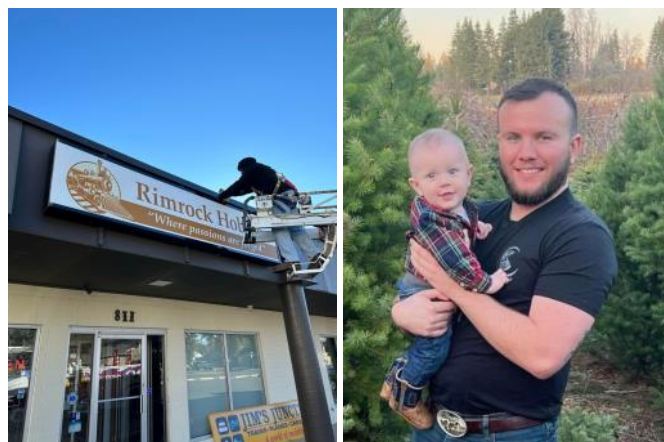
Left: New sign being installed at former Jim's Junction. Liam Dunne photos Right: Owner Liam Dunne with son Alec.
