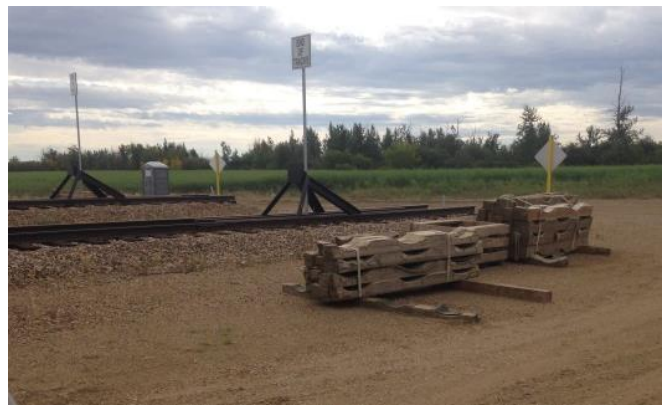
Saddles for 36" pipe banded and ready to return to the pipe plant.
