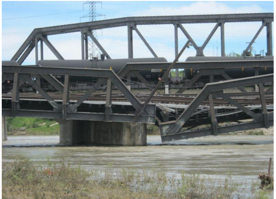
The Bonnybrook rail bridge on June 29 th a few days after a train derailed on it when flooding undermined the pier in the river. The bridge has since been dismantled. - Rob Badmington
